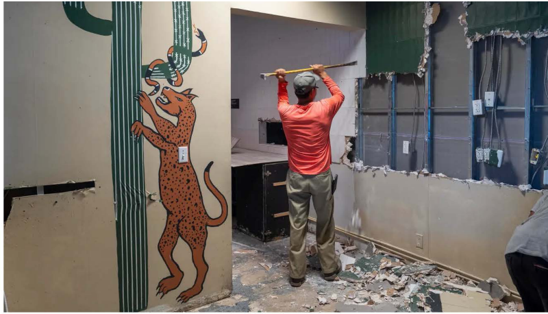
Workers begin demolition to reopen the Grandview Public Market food hall as a slimmed-down version with a stage and events and entertainment at the newly renamed Caroline Station in West Palm Beach, Florida, on October 16, 2025. GREG LOVETT/PALM BEACH POST
